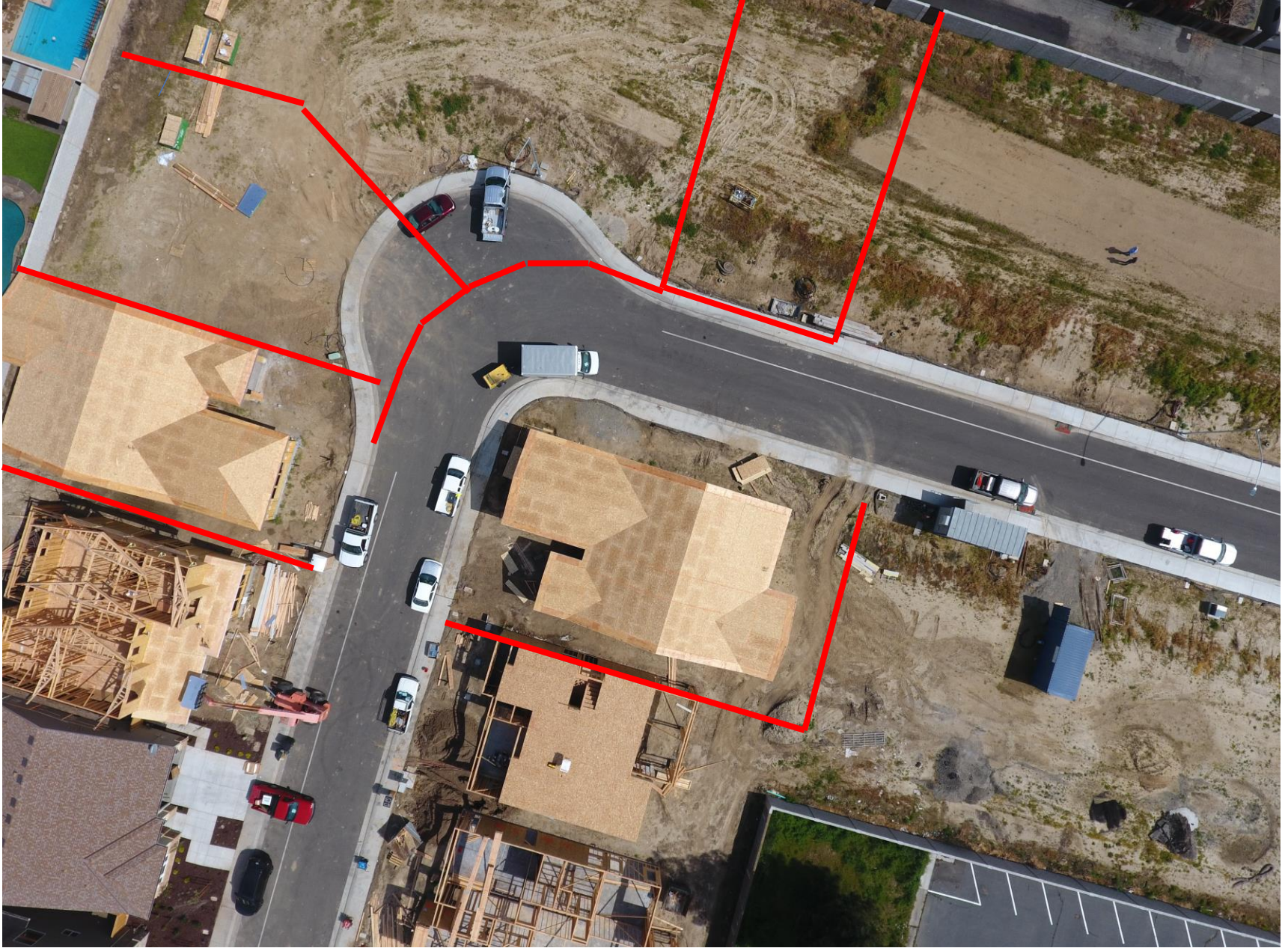
Lot yield without bumpout (1 lot less because there is not enough required frontage to meet code)
